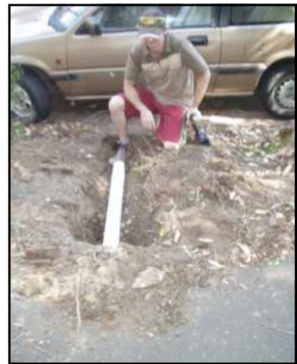
Replace the pipe leaving gaps at either end to slow down and absorb rain water at the ends
