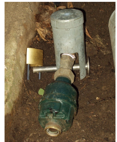
locked water meter
